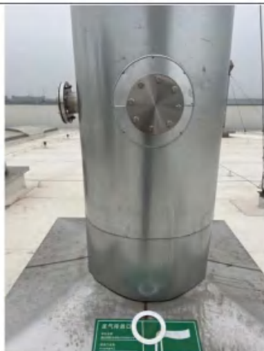
P10 排气筒出口监测口及环保标志牌
