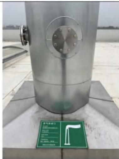
P11 排气筒出口监测口及环保标志牌
