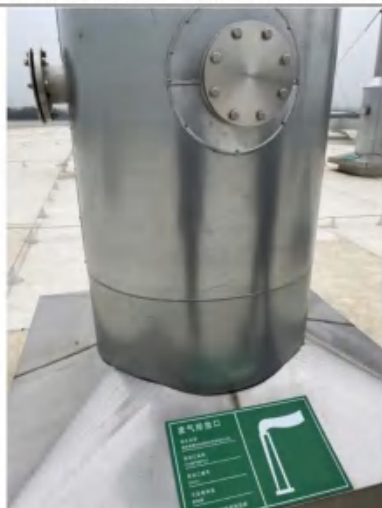
P15 排气筒出口监测口及环保标志牌
