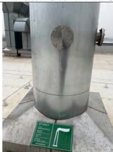
P14 排气筒出口监测口及环保标志牌
